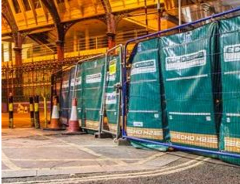
Figure 5 – Example of relocatable noise screens
