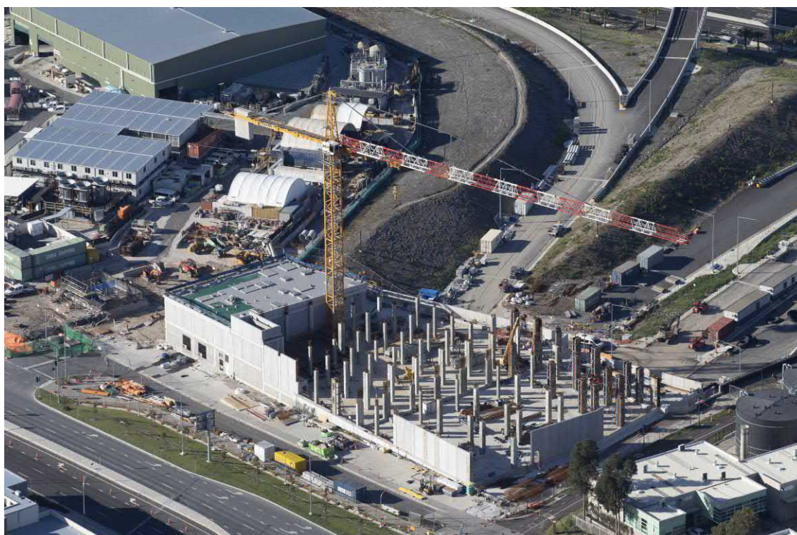
Figure 2-3 - Aerial view of the ventilation building at the Campbell Road site in March 2021
