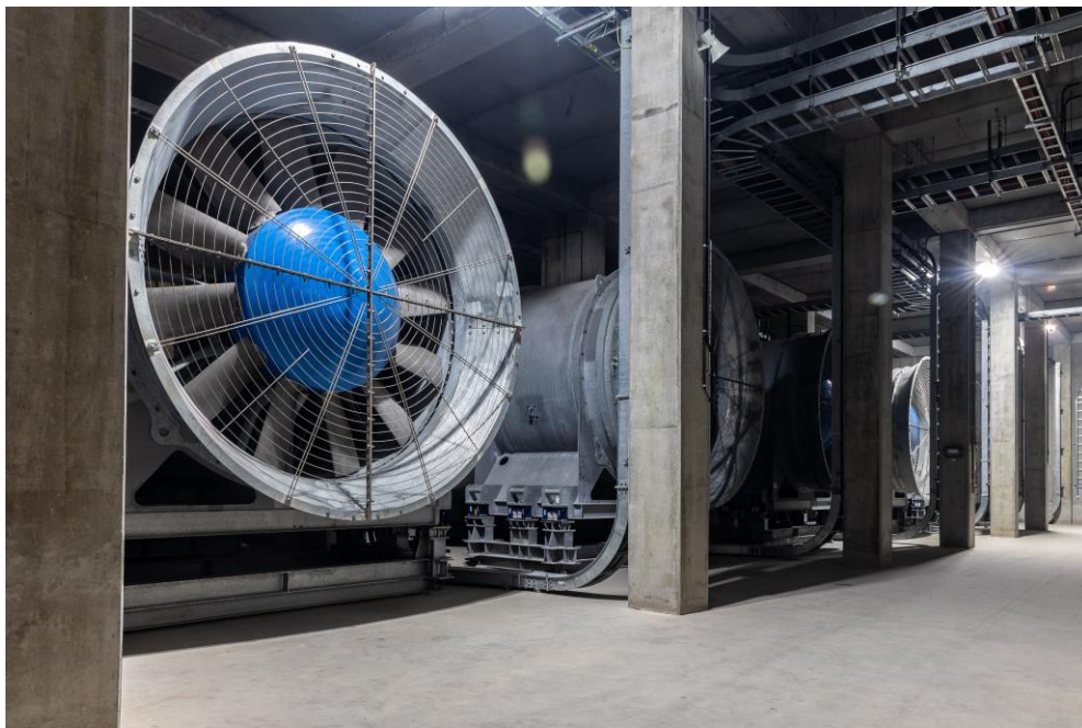
Figure 2-3 Ventilation building axial fans, St Peters, April 2022
