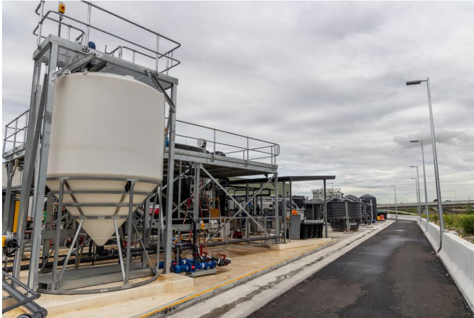
Figure 2-2 Operational water treatment plant, St Peters April 2022
