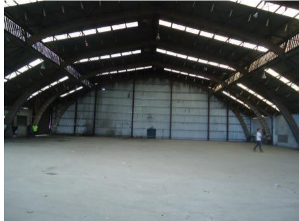
Plate 86 Interior of former Rudders Bond Store, showing open expanse created by arched form.
