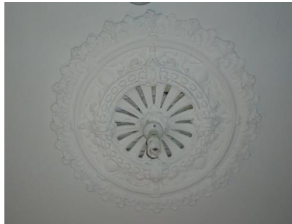
Plate 65 Interior of 44 Campbell Street. Ceiling rose in living room with lathe batons behind
