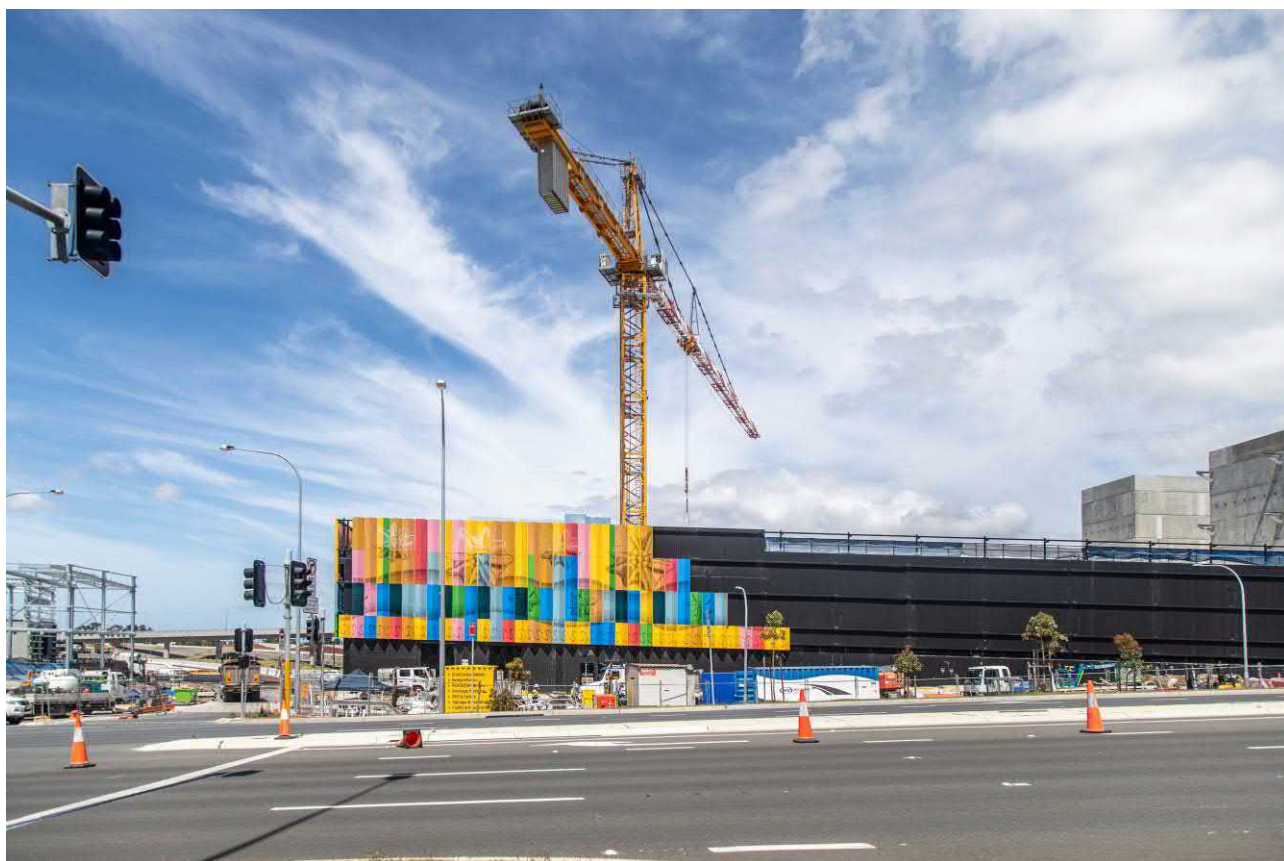
Figure 2-3 – Ventilation building artist cladding at the Campbell Road site in October 2021
